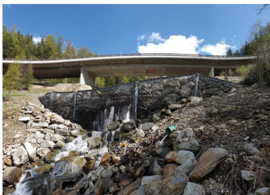
Pre-filled UX-180-H6 barrier, seen from downstream (Image: [G]).
