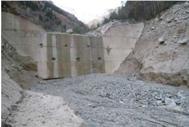
Figure 72. Deposition and scour at check dam n°11
