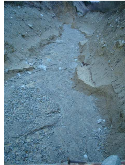
Figure 73. View from the brink of check dam n°11 on lateral erosion
