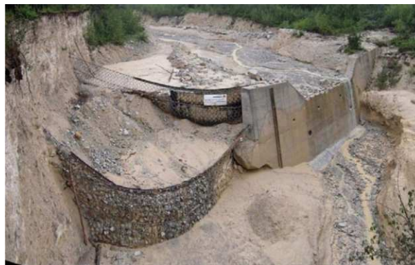
Figure 60. Lateral erosion and flexible ring net barrier at check dam n°25 [67]
