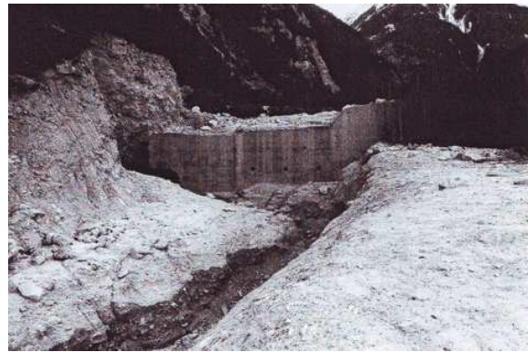
Figure 59. Overview of scour at check dam n°20 [52]
