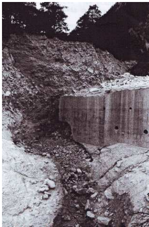
Figure 58. Lateral scour and destabilisation of check dam n°20 [52]
