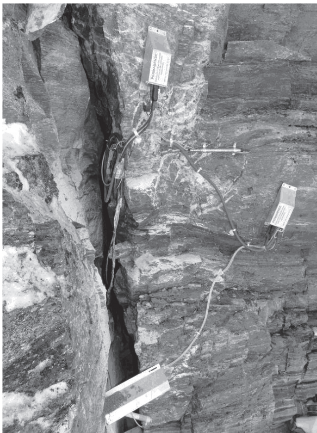
Figure 8. Installation site with multiple sensors: At the bottom, two crack meters measure dilatation. Within the cleft, potential water pressure and ice stress, as well as temperatures at different depths, are measured. The tube between the two nodes is the reference air pressure measurement.
